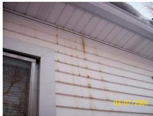
Stains from water leakage through siding weep holes
