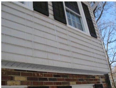
Water leaking through siding weep holes freezes when it hits cold air.
